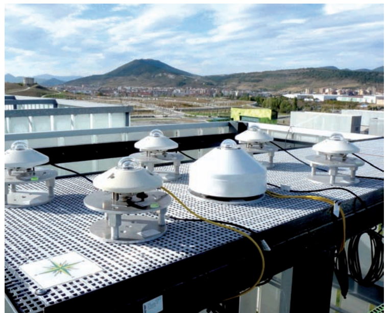
CENER Pyranometer calibration facilities
